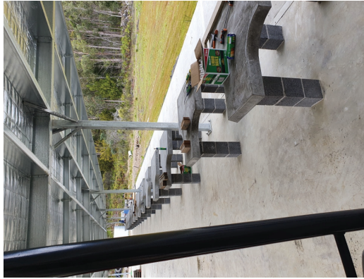
Sample Photo of Similar Firing Line Structure View to area under structure
